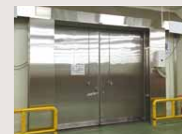
Cold storage Inside -25°C / Outside 5°C Size: 3,000mm (h) x 2,600mm (w) Door opening by Pull switch
